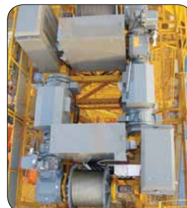
HOISTING & LUFFING GEAR
